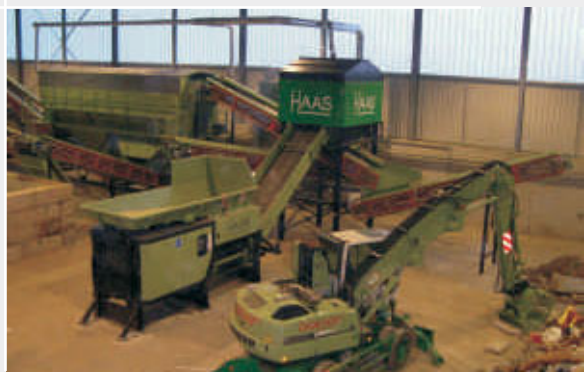
HAAS primary crusher, HDVV
